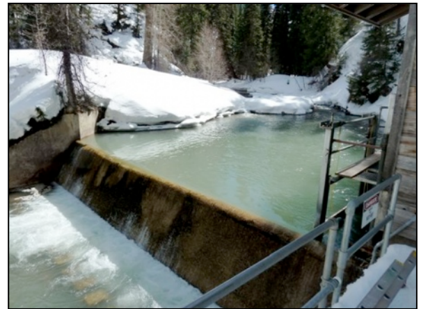
Figure 10. Through an intergovernmental agreement with the CWCB, Aspen has agreed to exercise its water rights in Castle Creek, including those for municipal diversions at the Midland Flume (above), in order to ensure that the CWCB’s 1976 minimum ISF water right (for 12 c.f.s.) is satisfied. (Brent Gardner-Smith, Aspen Journalism)
