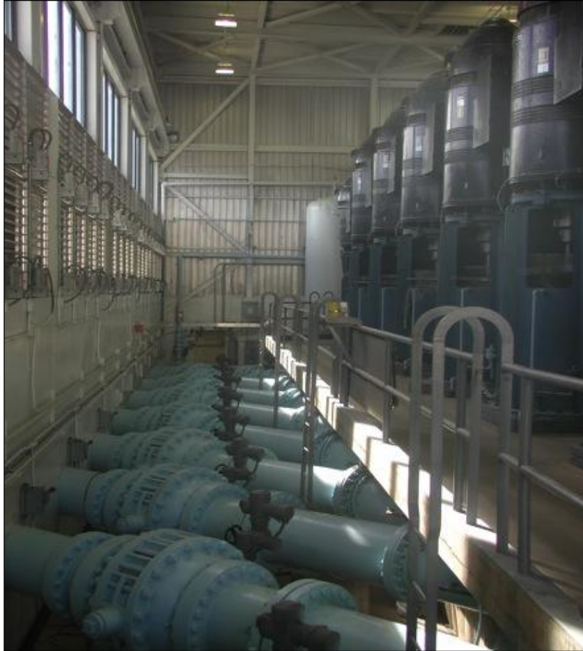
Otero Pumpstation (Colo. Springs Utilities)
