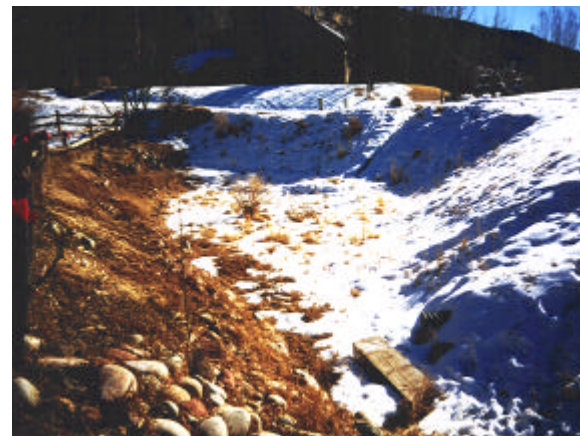
Figure 6: This sedimentation pond creates an opportunity for detention and water quality treatment by enlarging the pond and constructing a multi stage outlet.
