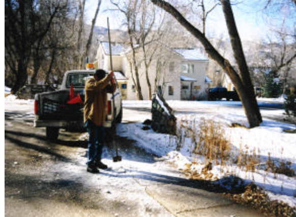
Figure 10: This is the Sample Point 3 outfall described in Figure 9. Icing and ponding will occur until new a storm drain is constructed. This intersection will flood in a major storm event.
