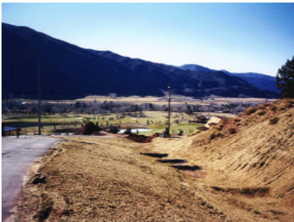
Figure 15: This newly constructed road and swale above the Roaring Fork Club is a good example of construction BMP's. The site is well stabilized using a series of check dams, along with seed and mulch, to prevent erosion of the construction site.
