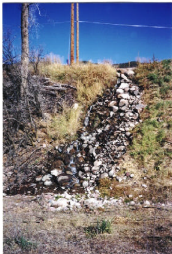
Figure 14: This steep run-down can carry a high sediment load into the Roaring Fork River. The slope should be stabilized against further erosion.
