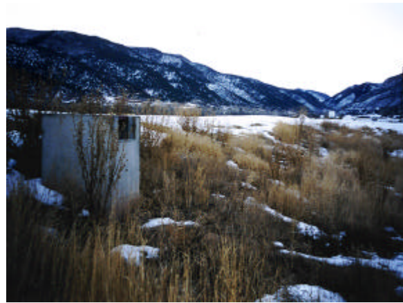
Figure 8: This retention pond at the Basalt High School manages stormwater runoff and treats stormwater runoff water quality. This outlet is designed to release the major storm event (100-year) before it can overtop the embankment. The grate should have been set below the level of the embankment.
