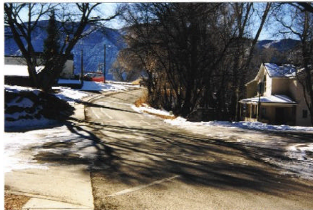
Figure 9: A total of 115 acres are tributary to this outfall for Sample Point 3. The existing culverts are inadequate to convey runoff from a major storm event and no formal outfall exists.
