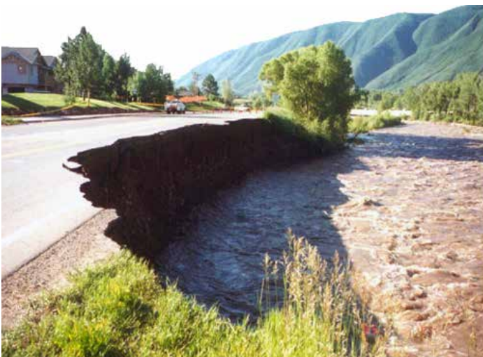
A section of Two Rivers Road was washed out.
