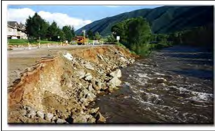
Figure 7. Eroded riverbank and road damage caused by high water near Basalt, 1995.
