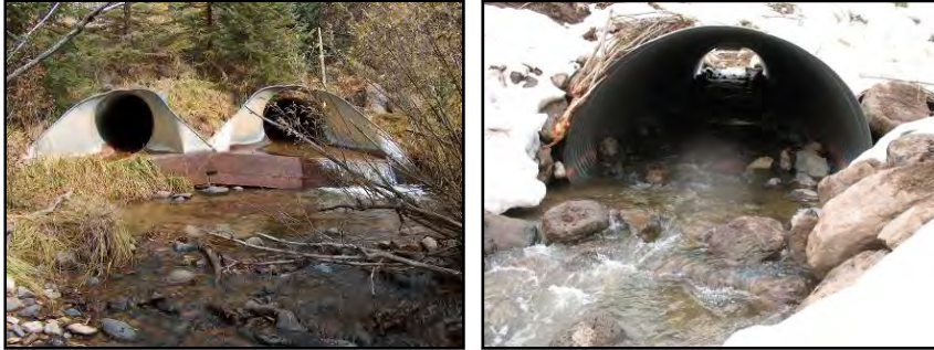
Figure 13. Before photo –These culverts were complete barriers to fish due to high velocity, no natural substrate, and location above the stream channel creating a jump barrier. After photo – This elliptical pipe dissipates stream velocity reducing the velocity barrier; pipe is embedded into the stream bottom at same grade as stream; and the bottom of the pipe is covered with gravels and cobbles creating a more natural substrate (Photo credit: Mark Weinhold, USFS).
